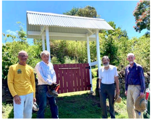
Volunteers Dan Gordon, John Ogg, Keith Barton, and Steve Mann stand in front of the new orchard gate which they constructed. Mahalo to our volunteer crew for their hard work week after week.
