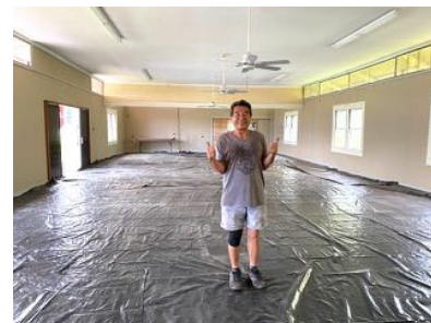
Contractor Glenn Uchimura giving "shakas" upon completion of the installation of the social hall panels.
